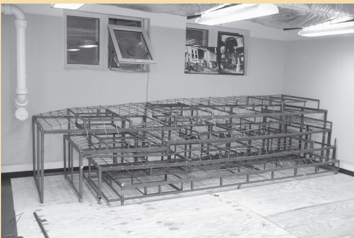
Figure 1. Tel substructure in LaSalle Banks multipurpose room, collapsed for storage, before addition of fiberglass layers. Photo by Erik Lindahl
